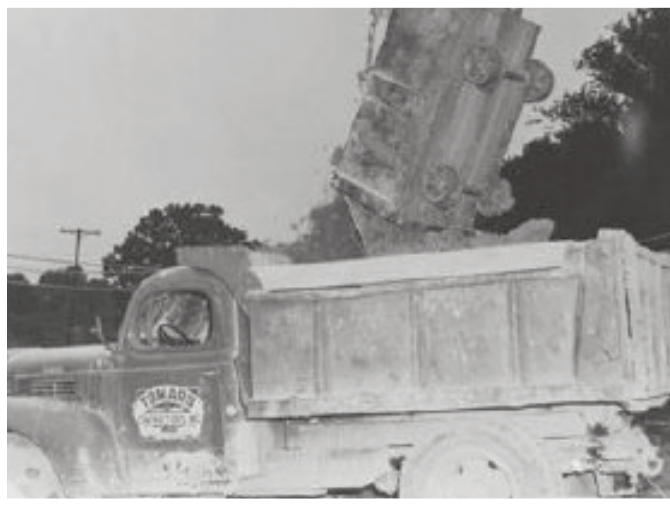
Muck car on a tunnel job involving then WUCA member Tomaro Contractors, Northwest Avenue tunnel in Racine, Wisconsin. Tomaro closed in the late 1980's after many decades of work in Wisconsin. (Photo from Operators Local 139)
